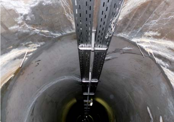
Leaky joint in the inspection walkway
