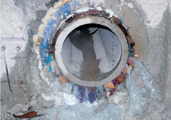
Leaky ring gap before injection
