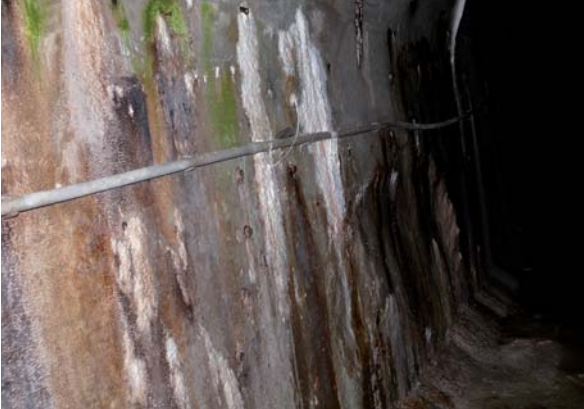
Leaky concrete in the inspection walkway
