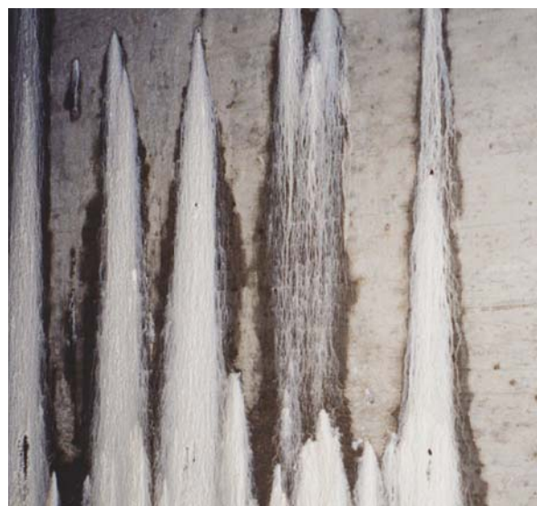
Leaking tunnel inner shell
