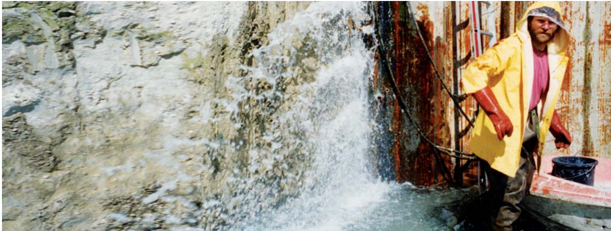
Leaking connection between the sheet pile wall and slurry wall
